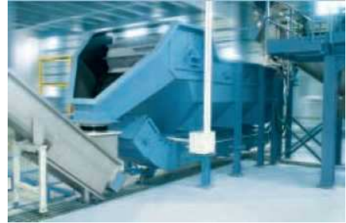
Flotation tank with scrape conveyor
