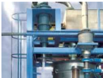
Part of a hydrocyclone plant
